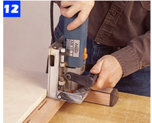
Lay out the plate slots in the table sides for attaching the bottom shelf. Use a straight board as a guide for the joiner.
